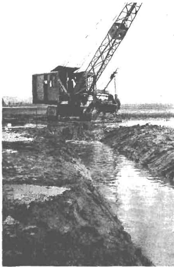
FIG. 84. Salt-marsh drainage operations with drag line mounted on timber mats to prevent sinking in mud. The bucket is about to cut into a breeding pool which will be drained into ditch in foreground. (Photograph by H. F. Gray.)
